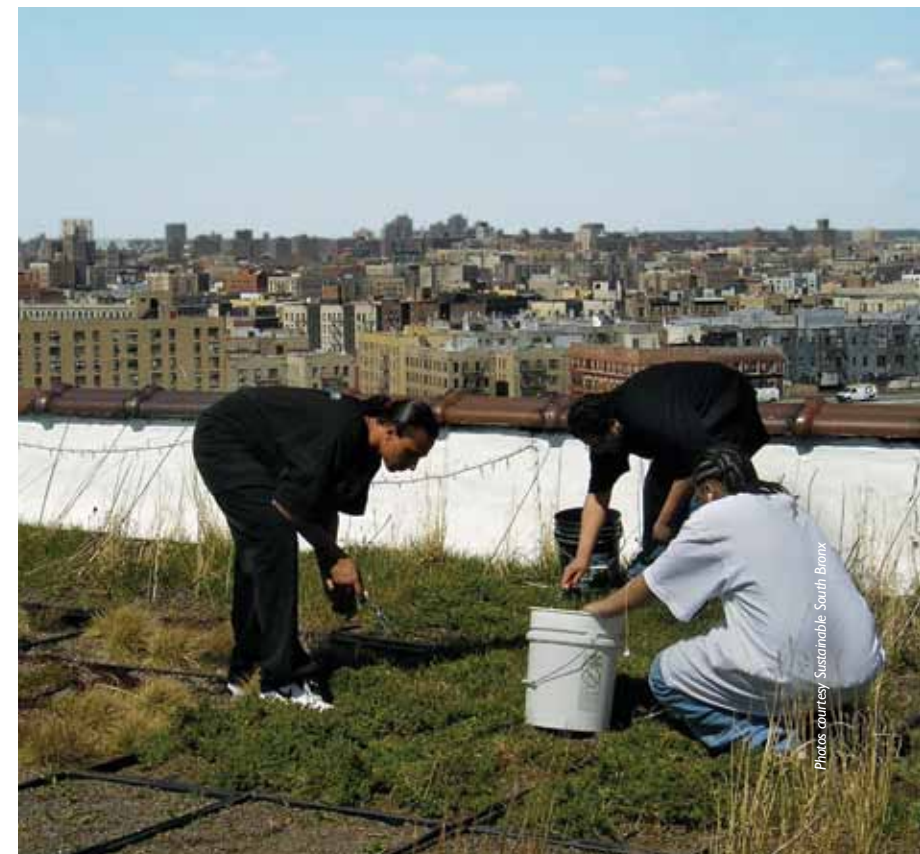
Green collar workers from Sustainable South Bronx turn a rooftop into a green roof.
